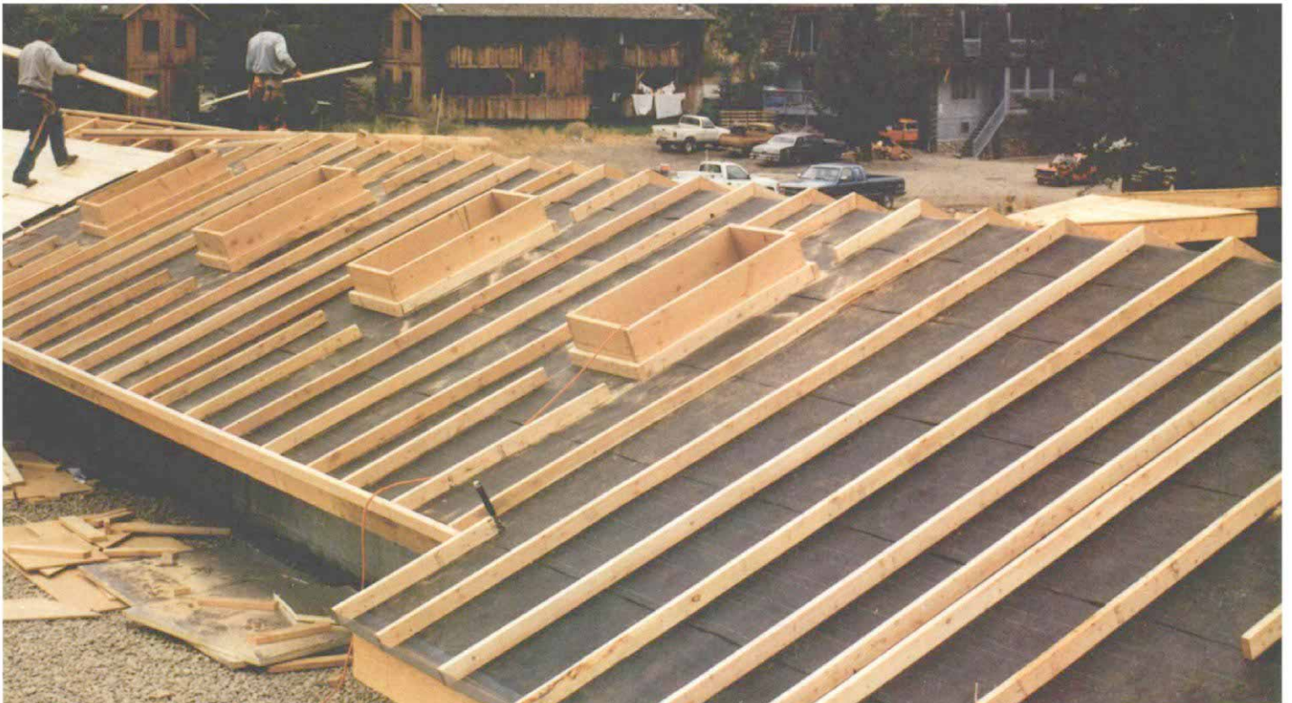
In this application of a cold roof, the sleepers extend several inches past the fascia of the underlying roof to form a protected vent area. Screening (just visible in the foreground of the photo above) has been stapled in place to keep bugs and birds from invading the roof later on.
