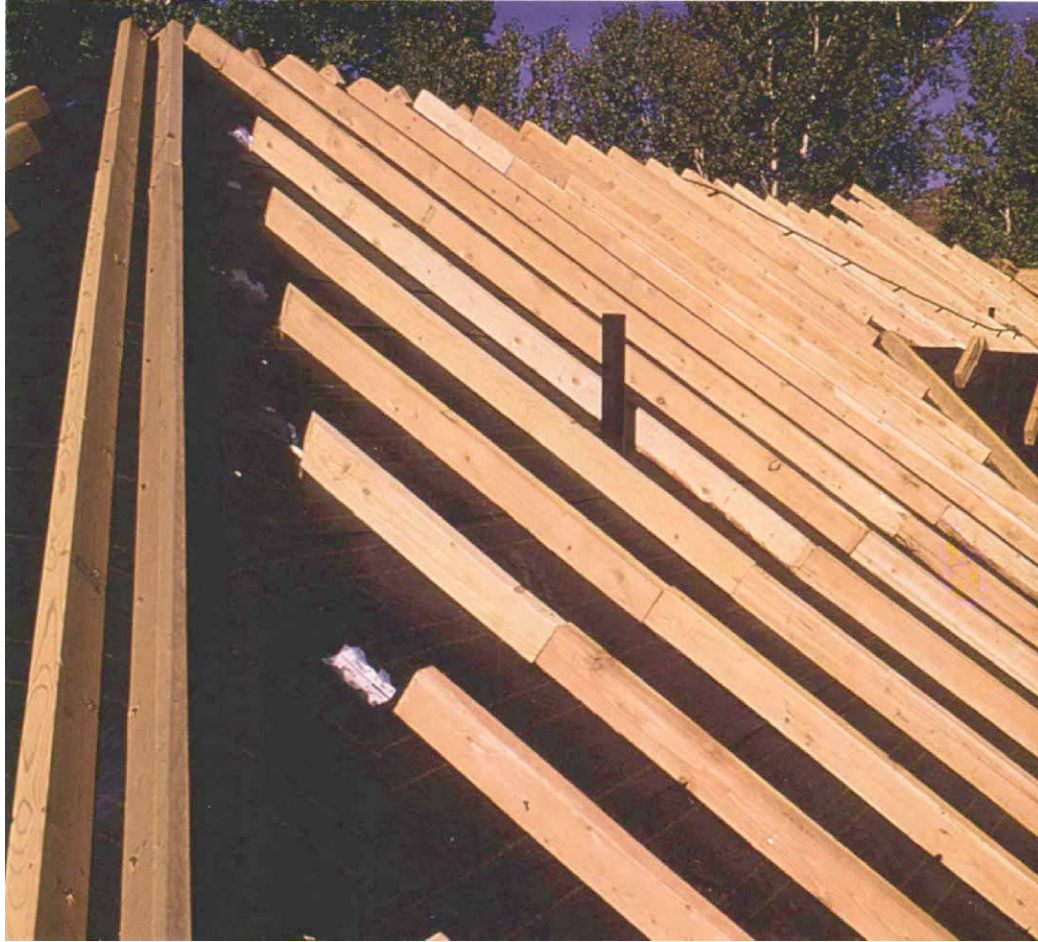
The sleepers on adjoining roof planes at hips and valleys should be oriented to channel air upward. Nothing should obstruct the flow of air from soffit to ridge.
