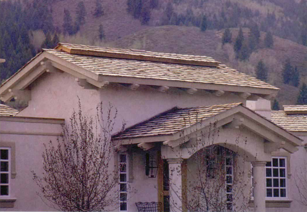
The Boston ridge (photo above) used for a cold roof is a site-built variation of the standard ridge vent, but with an overhang that prevents it from clogging with snow. Two methods for framing the vent are shown in the drawings below.
